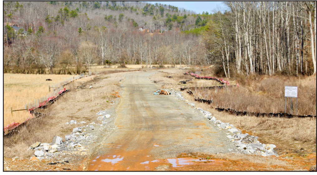
Much work has already been done to cut in the new Young Harris Bypass, with construction slated to resume next week. Photo by Shawn Jarrard
